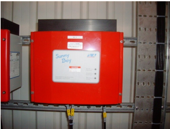
Figure 2 - Typical inverter under test
