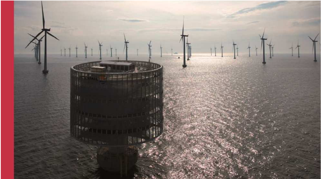
Siemens offshore substation, Lillgrund, Sweden
